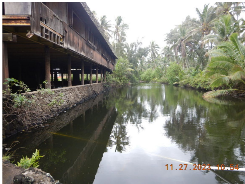
Photograph 4: View, facing south, of the Weuweu kawai iki fishpond. Note that the building pictured on the left is one of the buildings that will be undergoing construction. Photograph taken by Randee Tubal on November 27, 2023.
