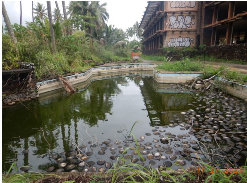
Photograph 9: View, facing north, of one of the three swimming pools on Site. Note that the pool is situated between the resort and the fishpond (refer to Image 3). Photograph taken by Bobbie Teixeira on November 27, 2023.
