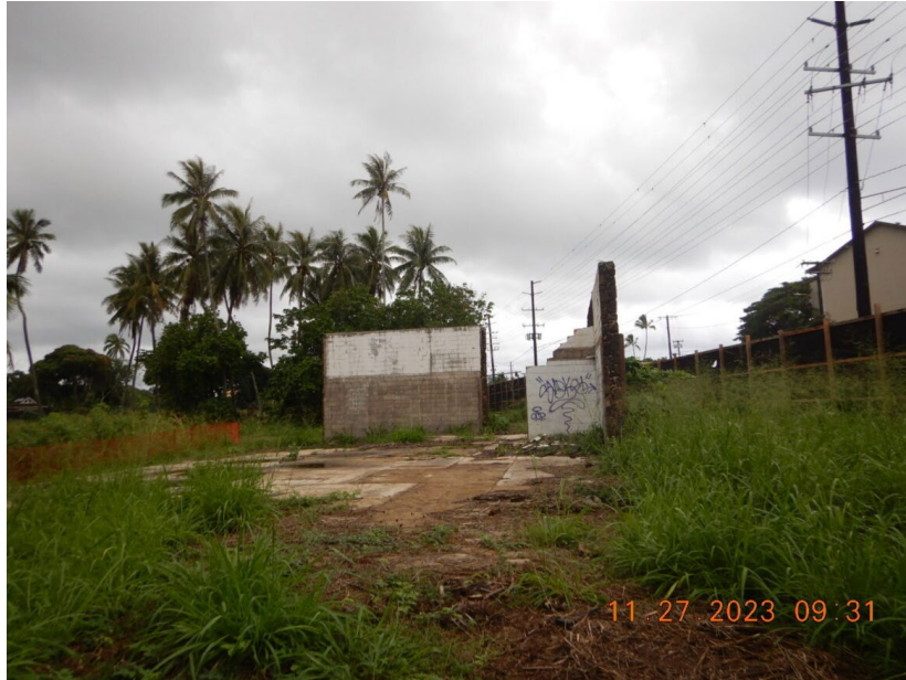
Photograph 21: View of the walls on Parcel 7, slated for demolition. Photograph taken by Randee Tubal on November 27, 2023.
