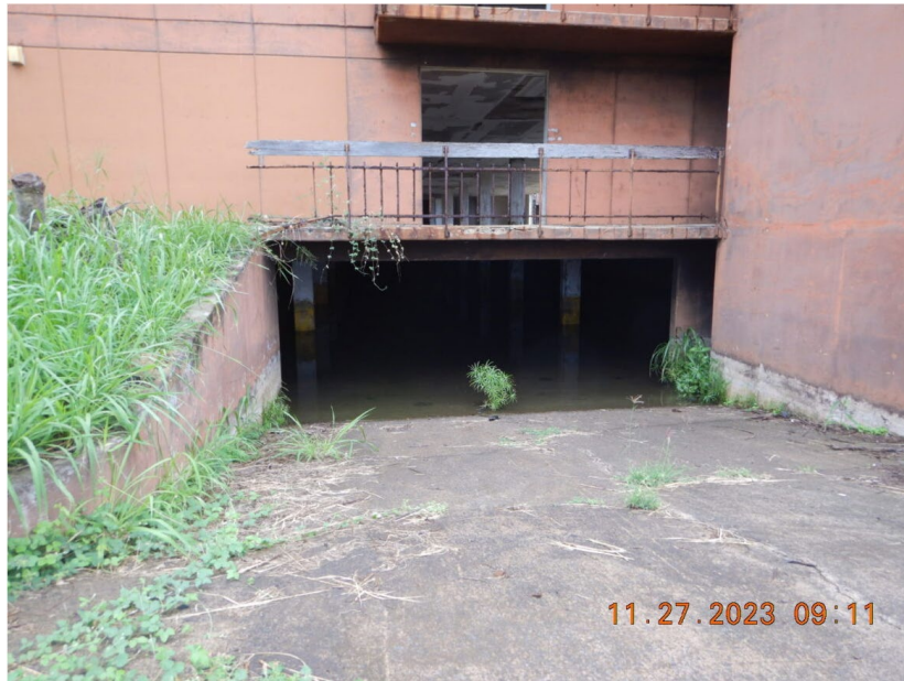
Photograph 7: View, facing north, of Building 1. Note the standing water located in the underground parking structure. Photograph taken by Randee Tubal on November 27, 2023.
