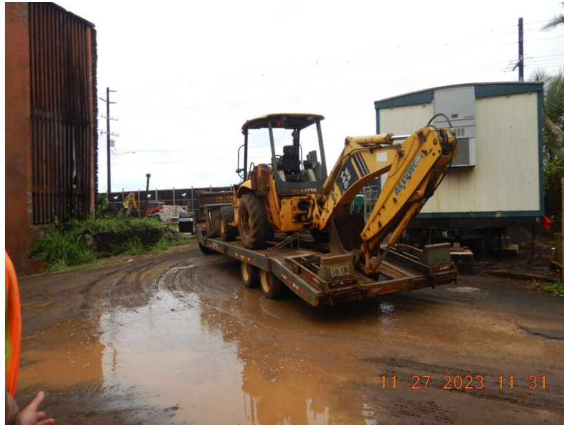
Photograph 15: View, facing northwest, of heavy equipment being trucked onto the Site. Photograph taken by Rande Tubal on November 27, 2023.
