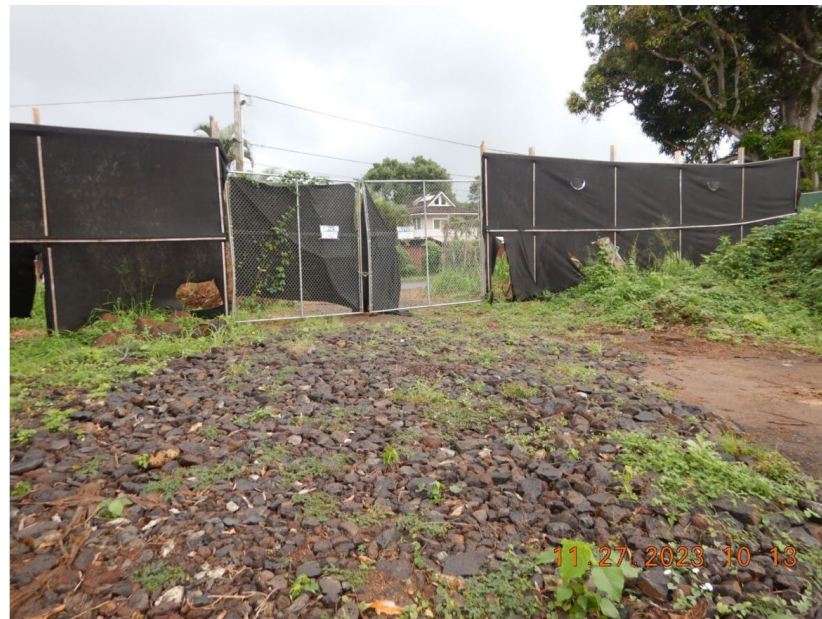
Photograph 12: View, facing northwest, of the third construction entrance located off Apana Road. Photograph taken by Rande Tubal on November 27, 2023.
