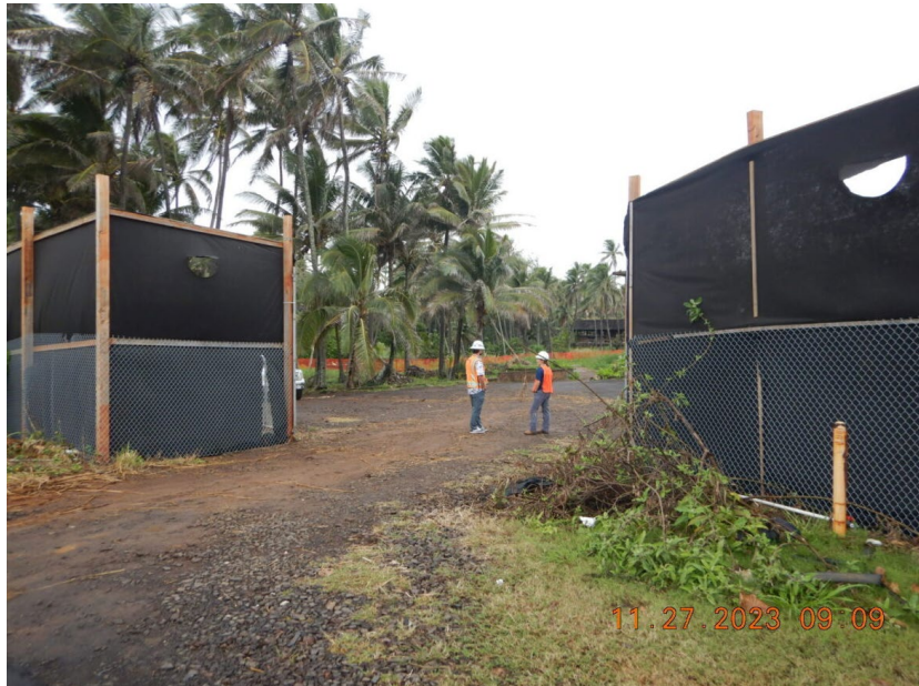
Photograph 1: View of the front entrance of the Coco Palms Resort Construction Site. This entrance is located off Kuamoo Road. Photograph taken by Randee Tubal on November 27, 2023.
