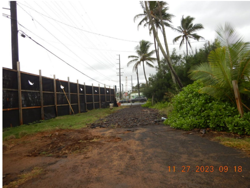
Photograph 11: View, facing south, of the second construction entrance located off Kuamoo Road. This entrance is approximately 20 m east of the entrance pictured in Photograph 1. Kuhio Highway is located on the other side of the dust screen. Photograph taken by Rande Tubal on November 27, 2023.
