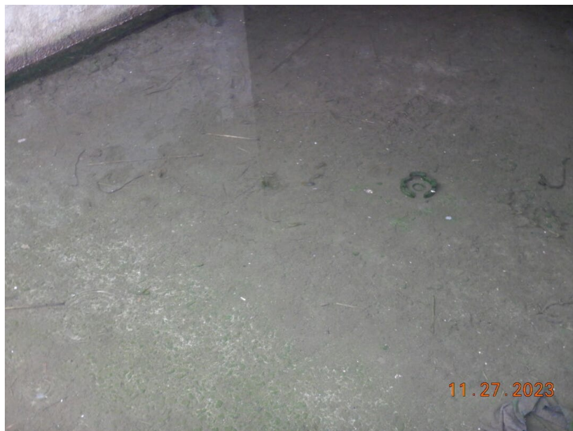
Photograph 8: Close up view of the standing water located in the underground parking structure beneath Building 1 (see Image 3). Photograph taken by Bobbie Teixeira on November 27, 2023.
